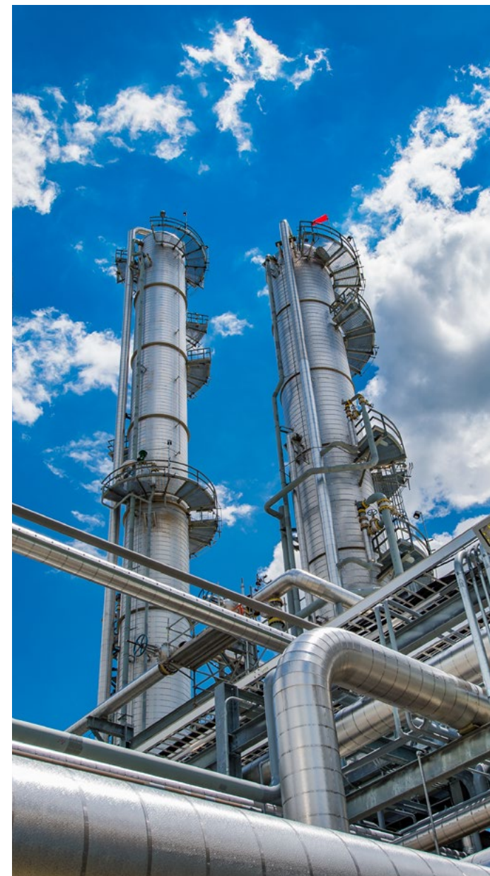
Our natural gas facility in Hopedale, Ohio.
